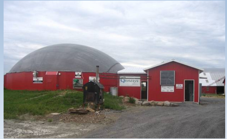
Terryland Farm Digester
