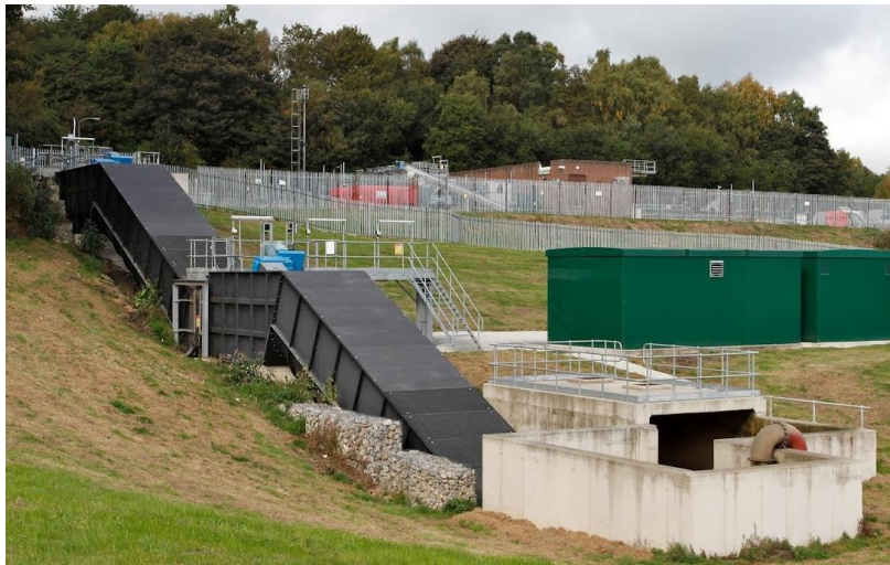
Figure 2.9: Yorkshire Water's Esholt wastewater treatment ASG hydropower plant [89].
