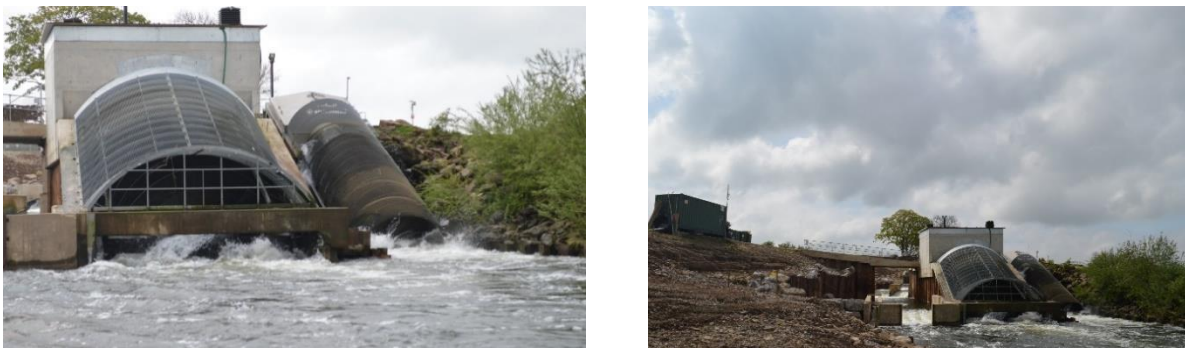
Figure 2.17: Linton Lock multi-ASG powerplant.
